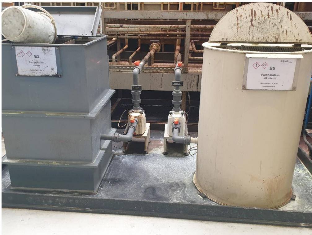
Abb. 7: Pumpstationen, pumpt Abwasser in Abwasser-Tank, Absaugung 18.000 cbm/h
